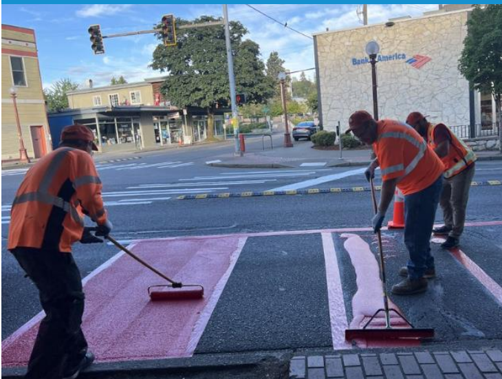
Transit spot improvements and design of improvements on high-ridership bus routes such as on Rainier Ave S and Beacon Ave S
