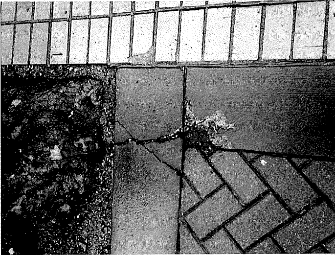
Cracked Pavers around several of the trees and bollards.
