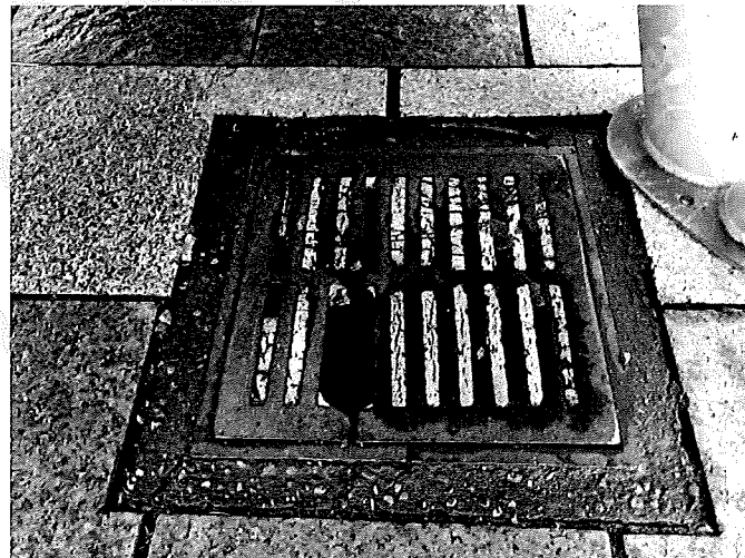
Drain grate is clogged and damaged.
