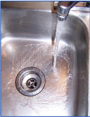
Toilets, Sinks, Showers, Washing Machines
