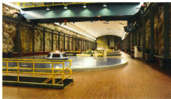
In 2015, staff repaired and returned Boundary Dam's generator unit 53 to service before the peak generation season on the Pend Oreille River in half the repair time expected and $1 million under budget. The unit went down in 2013.
