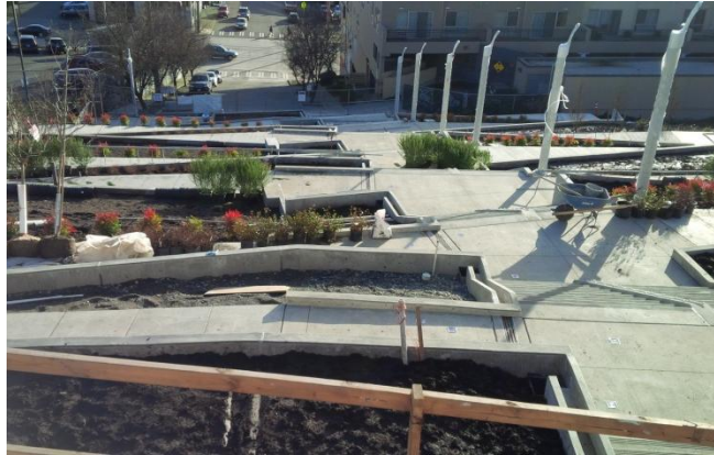
In 2015, the concrete stairs and ramps were poured for the 10 th Ave S Hillclimb.
