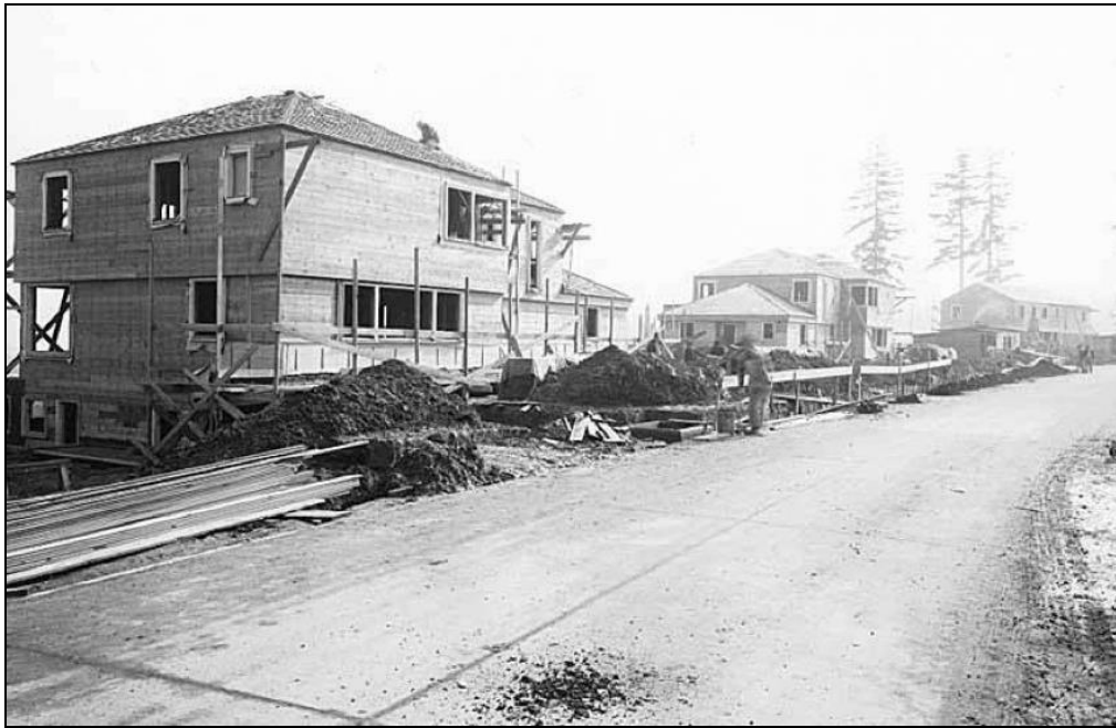
Construction of the Officer's Quarters. Photo Source: University of Washington Special Collections, Image No. SEA2801.
