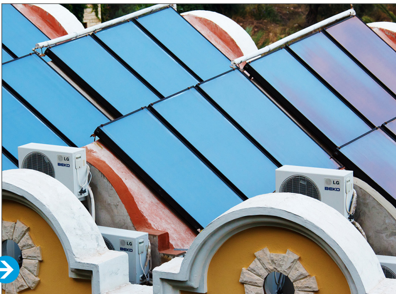
A roof-top installation of flat-plate solar thermal collectors. The system captures medium-temperature heat and circulates it to residential or commercial buildings to meet demand for space heat and hot water.
