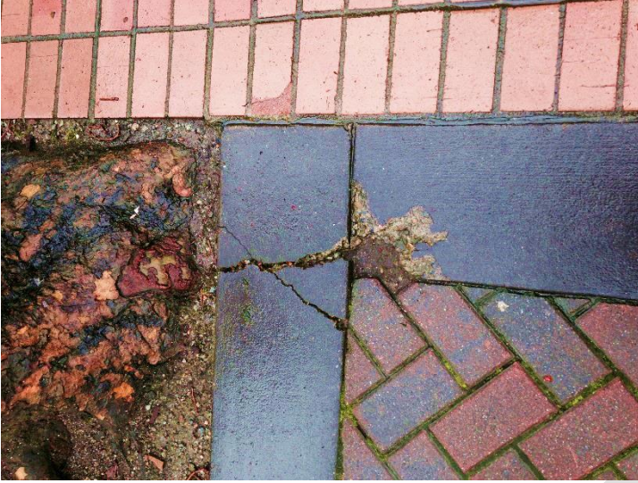
Cracked Pavers around several of the trees and bollards.
