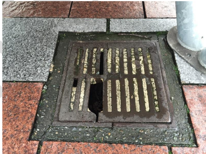
Drain grate is clogged and damaged.
