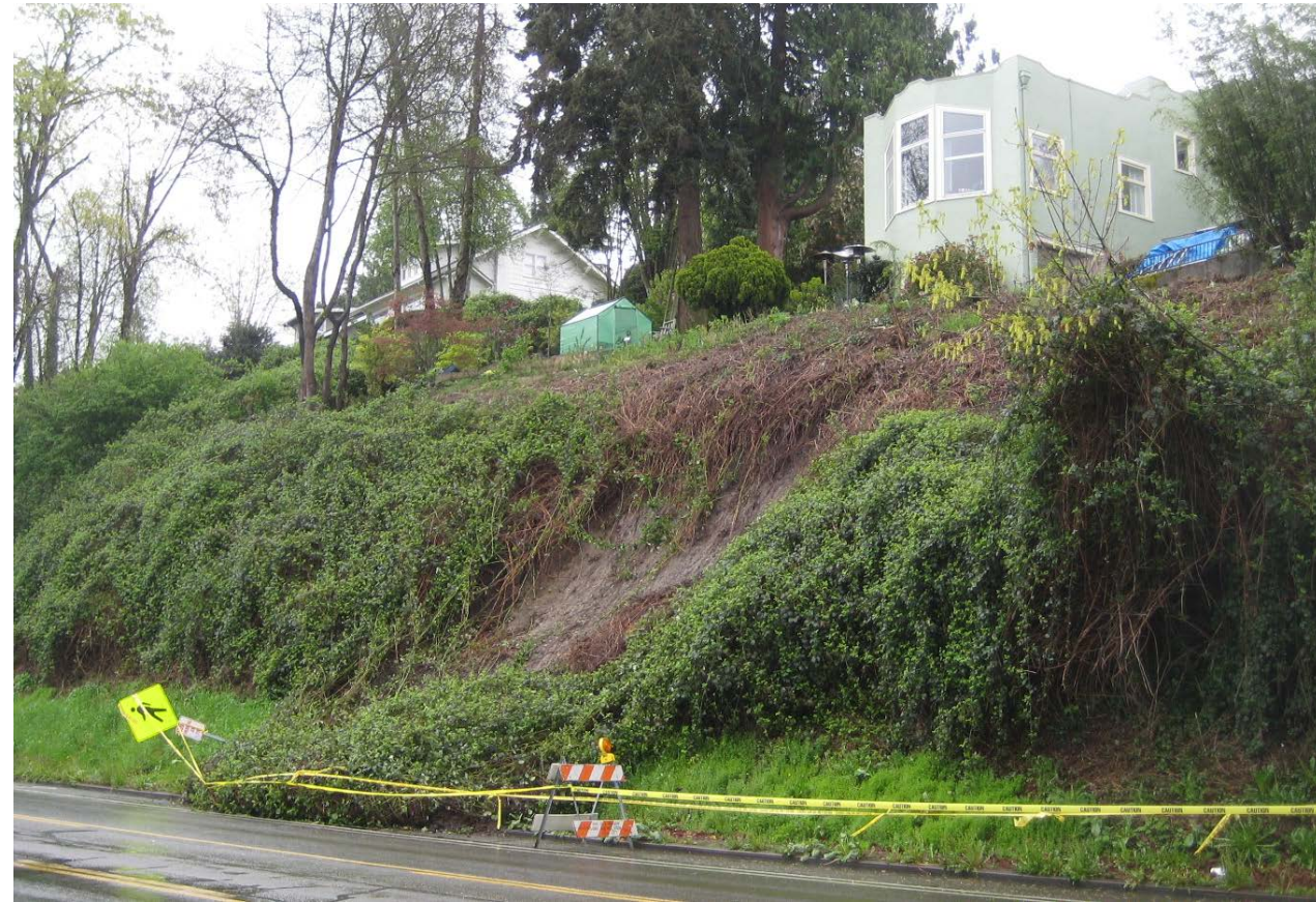
Unstable slope areas
