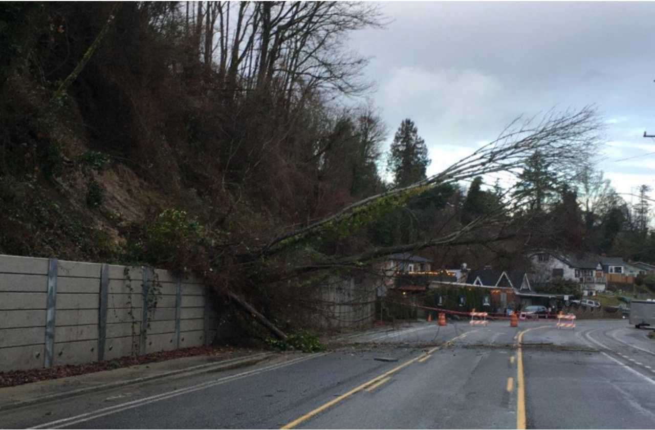
Debris flow from adjacent slope on sidewalk
