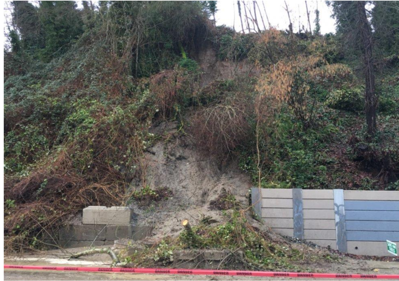
Unstable slope areas
