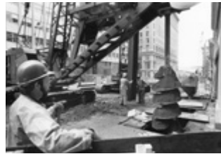
▲ Removing dirt from a hole for a soldier pile on Third Avenue near Yesler Way. April 30, 1987 Credit: MOHAI, Seattle Post-Intelligencer Collection
