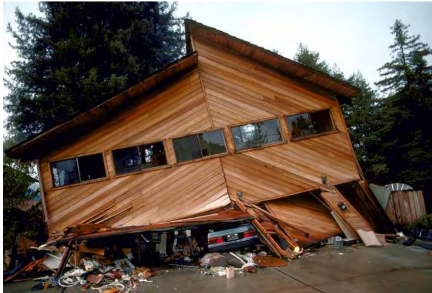
Figure 5-8. Home Damage Due to Inadequate Cripple Walls
