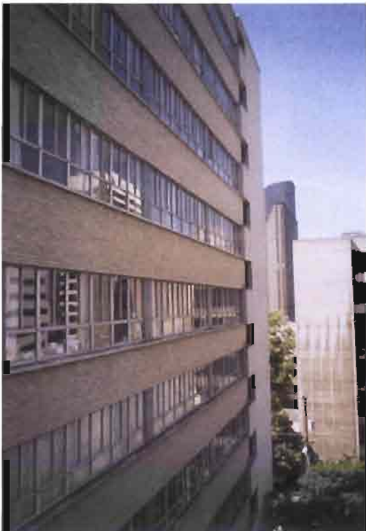
Figure 18A. Below left, partial view of the north facade of the 1954-1955 West Wing addition. 18B. Below right, view of the West Wing south and partial east facades.
