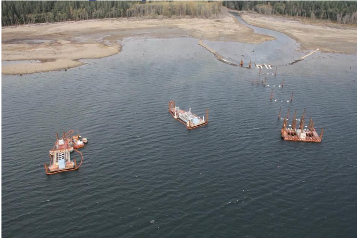
Outlet Channel (Top); Discharge Dike (Middle) PP2 – PP1 – MLTPP (L to R);
