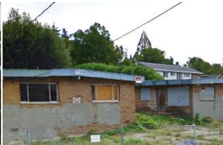
Apartment buildings in Lake City neighborhood. Vacant for over 7 years. Located in a commercial zone.
