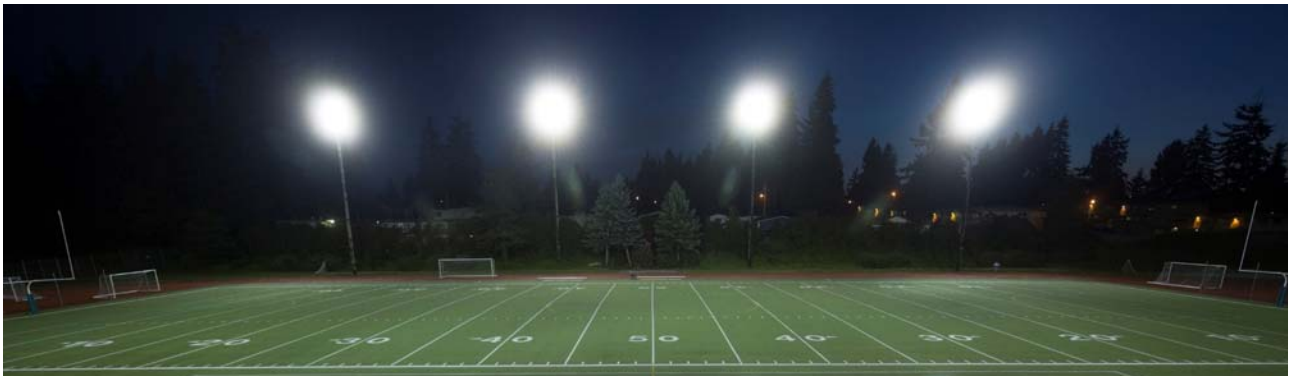
Example Un-shielded Metal Halide fixtures
