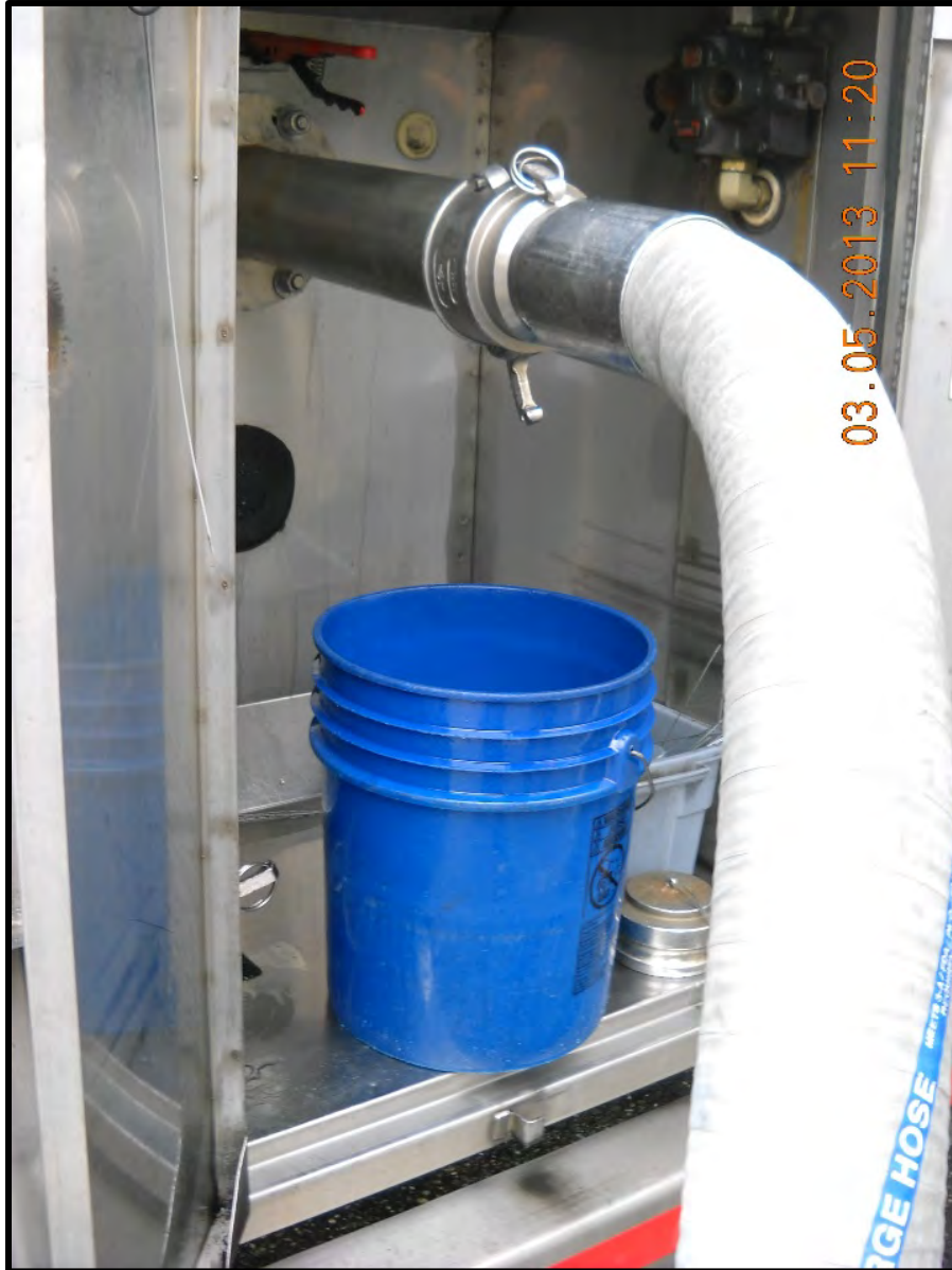
Figure 8. Temporary Containment Device Placed Under a Hose Connection.
