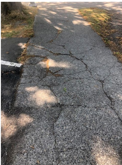
Extreme cracking on a segment of sidewalk near Lighthouse for the Blind.
