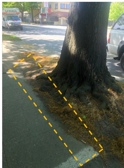
Street tree root structure encroaching on sidewalk near Lighthouse for the Blind.
