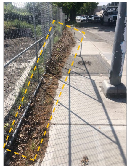
Street debris encroaching on pedestrian right of way on sidewalk near Lighthouse for the Blind.
