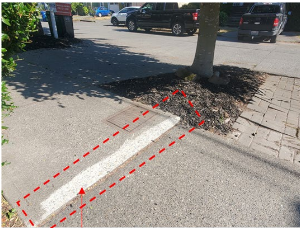
Example of a bevel : Edge of sidewalk was ground down so it matches the height of the neighboring concrete panel.
