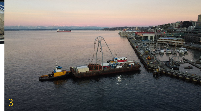
1. Jan 15, 2024: Submarine Cable pulling rig on Pier 66 2 and 3. Jan 15, 2024: Submarine Cable lay at Pier 66
