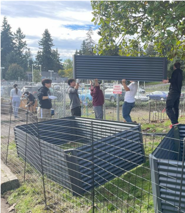
Lake City high school youth and their families install a new fence and several raised beds for their garden.
