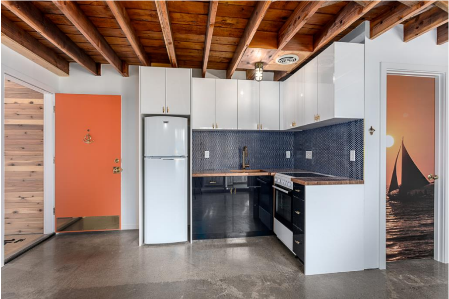
Full restoration of a MCM house in West Seattle - 2,200 sqft home - renovation down to stud.
