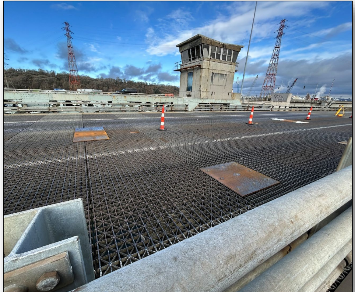
Phase II emergency repairs in April and May will replace 10 failing steel deck grid panels covered by steel plates since temporary repairs were completed in March.
