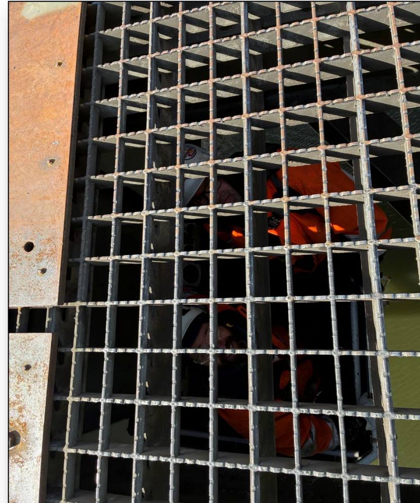
Repairs completed over five days in March 2026 addressed fractures in steel deck grates.
