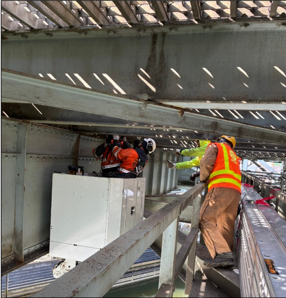
WSDOT maintenance crews repaired the northbound SR 99 First Avenue South Bridge from above and below in March 2026.
