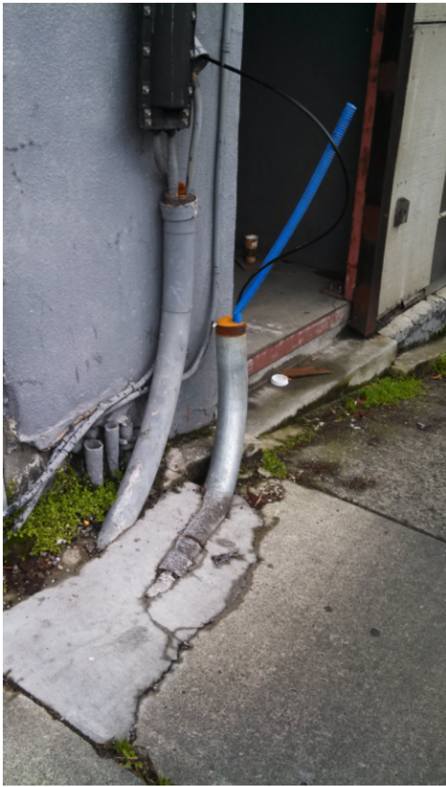
Comm conduit to building
