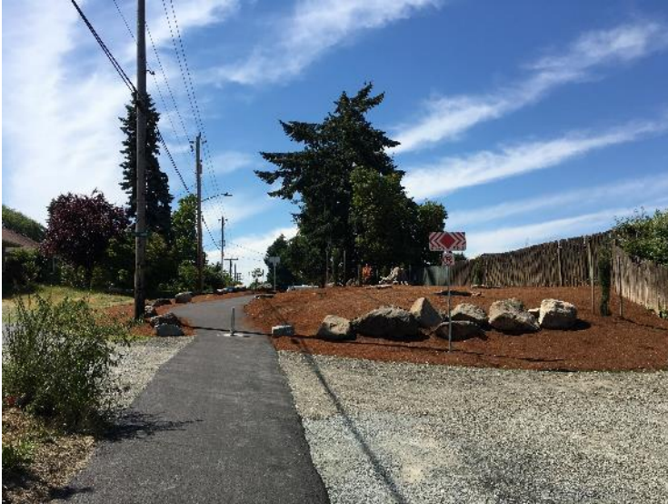
At-grade asphalt: Ashworth Ave N – N 122 nd St to N 125 th St
