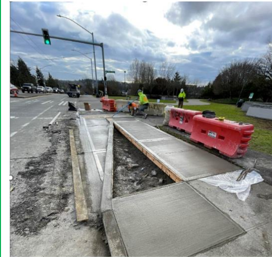
Construction crews paving new southbound bike ramp at I-90 Trail. Photo SDOT.
