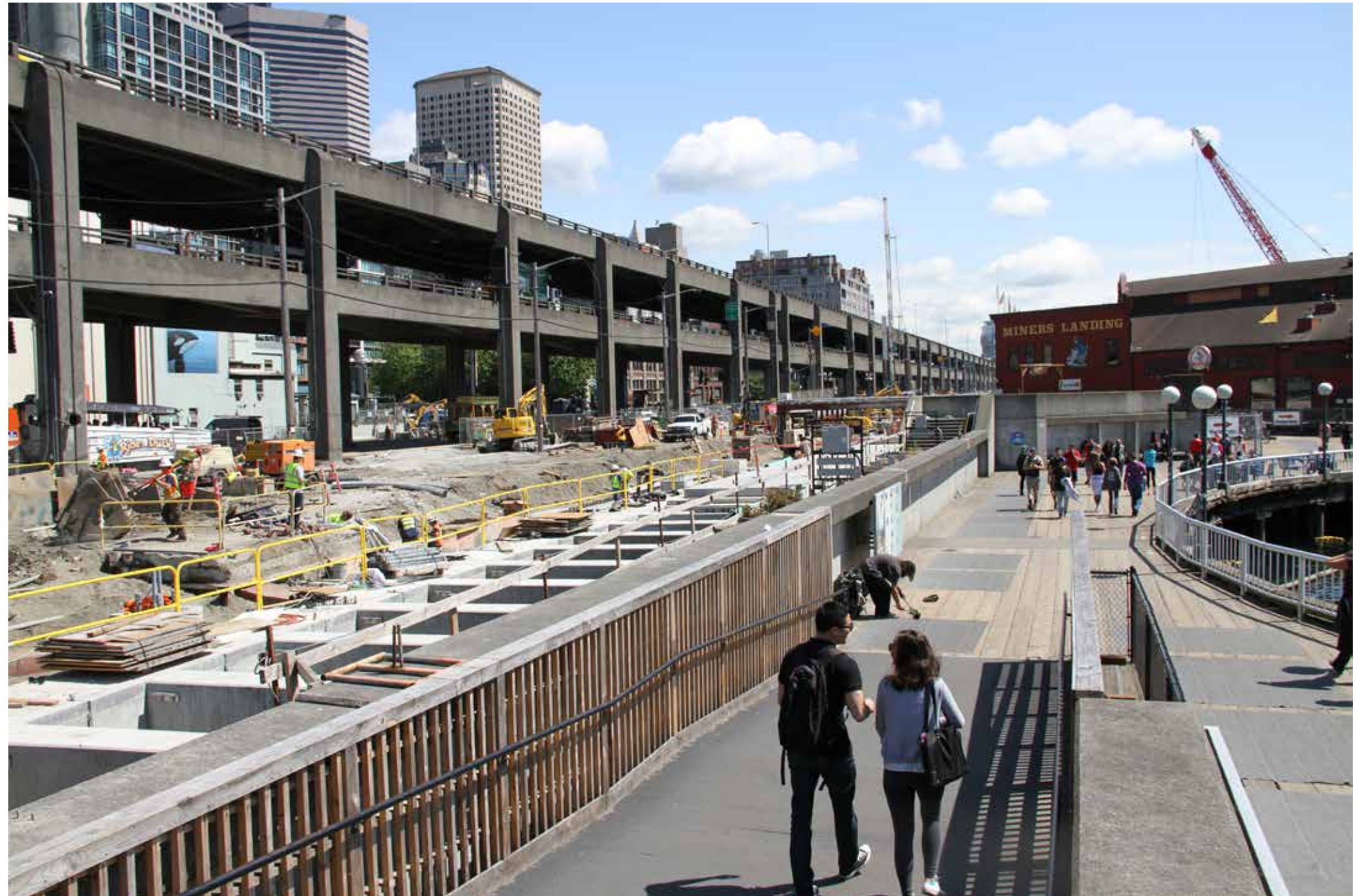
Replacement of the seawall is the first step toward realizing a new waterfront public space.
