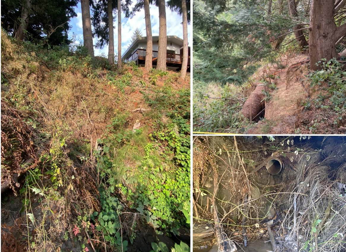
2022 – unstable slope & failing culvert
