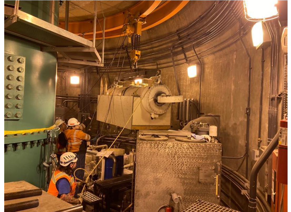
The cylinder is lowered into a custom-built cradle, and removed from pier house using internal crane rails
