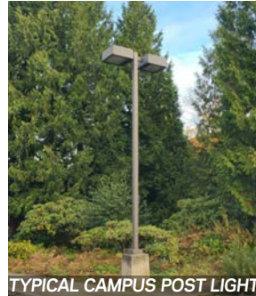
TYPICAL CAMPUS POST LIGHT
