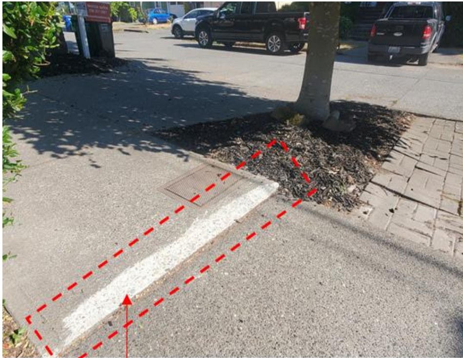
Example of a bevel : Edge of sidewalk was ground down to match the height of the neighboring concrete panel.
