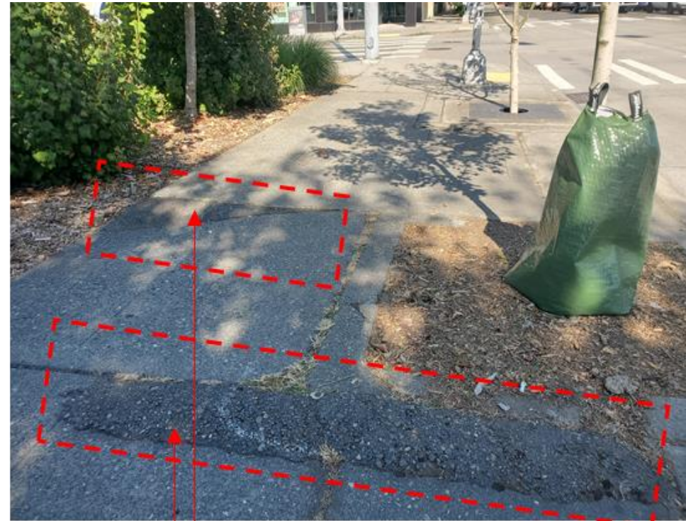
Example of shims : Asphalt was added to match the height of the neighboring concrete panel.
