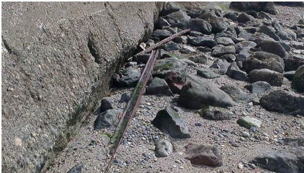
Figure 3. Corroded steel rails and failed top waler which historically held tie back anchors. Also note scour of sediments adjacent to concrete footing.
