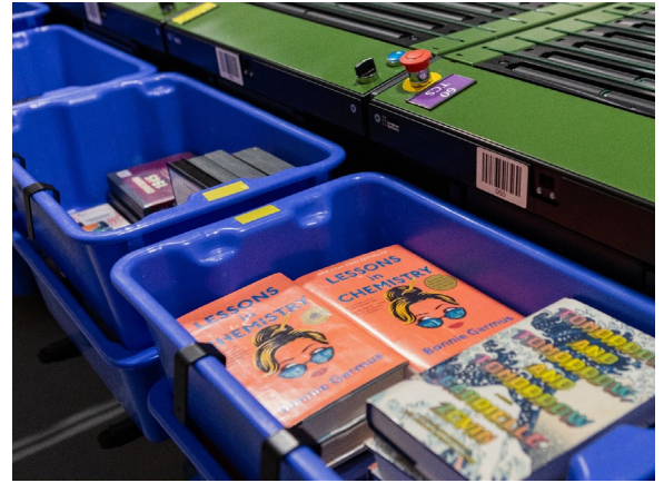
New Automated Materials Handling System at the Maintenance and Operations Center
