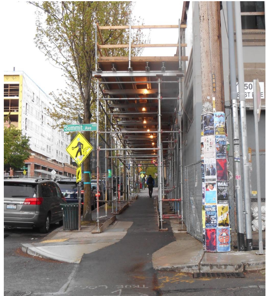
Scaffolding with detectable baseboard
