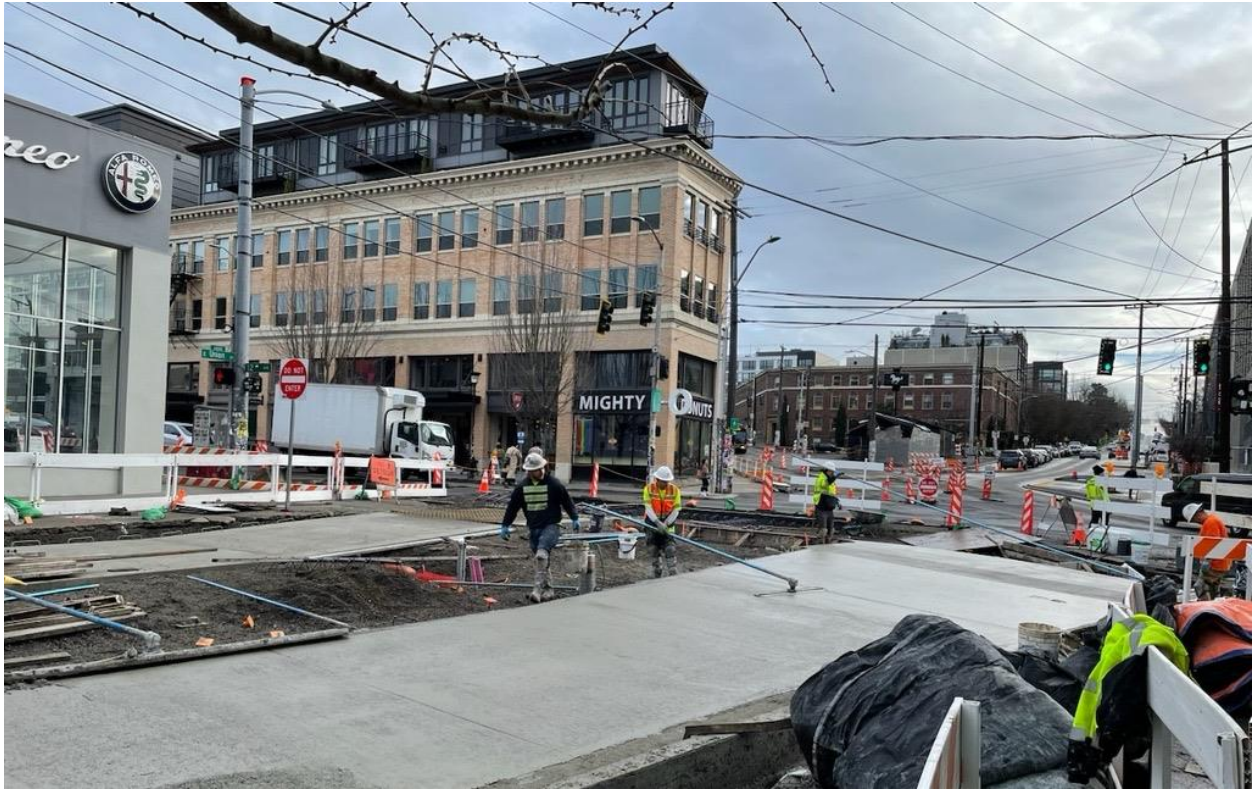
Program 18 – Work on Madison St as part of the Madison RapidRide G Line project.
