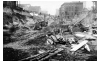
▲ Third Avenue looking south from Madison during regrade work. March 28, 1907 Credit: Seattle Municipal Archives
