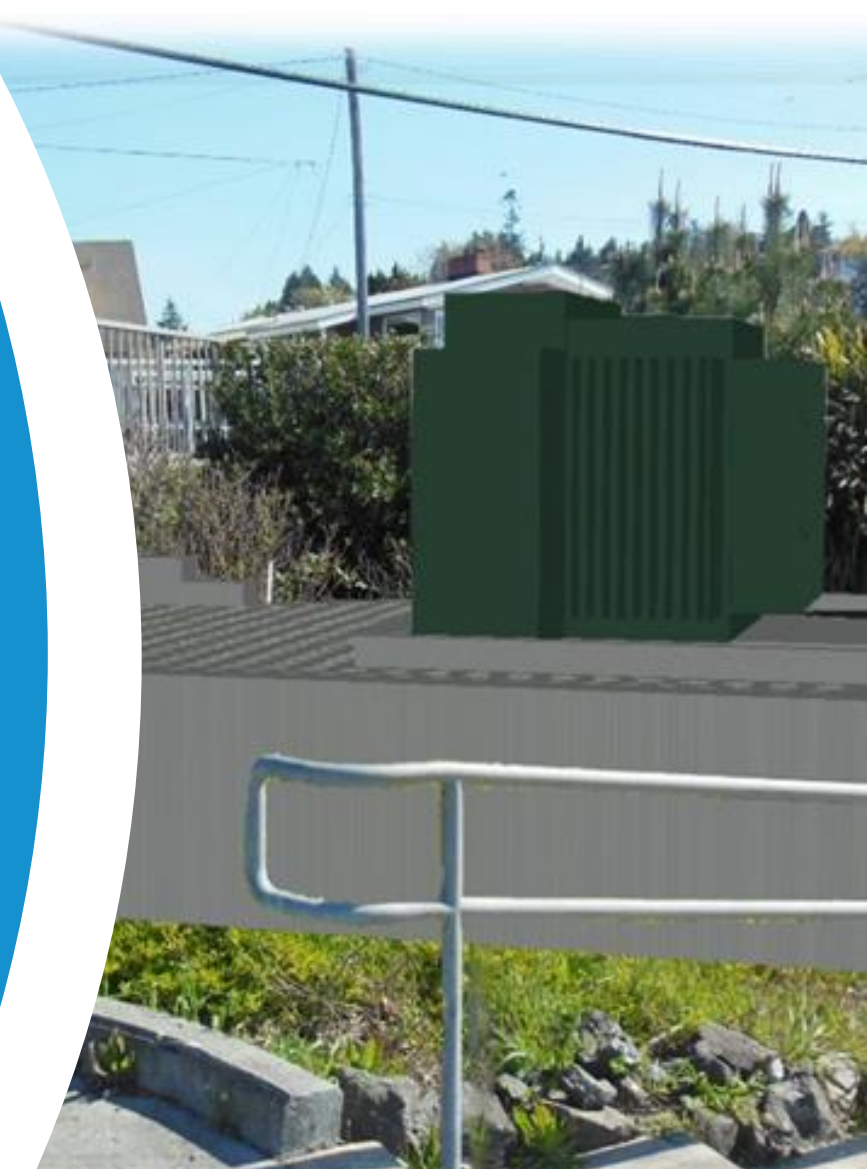
King County Alki Transformer
