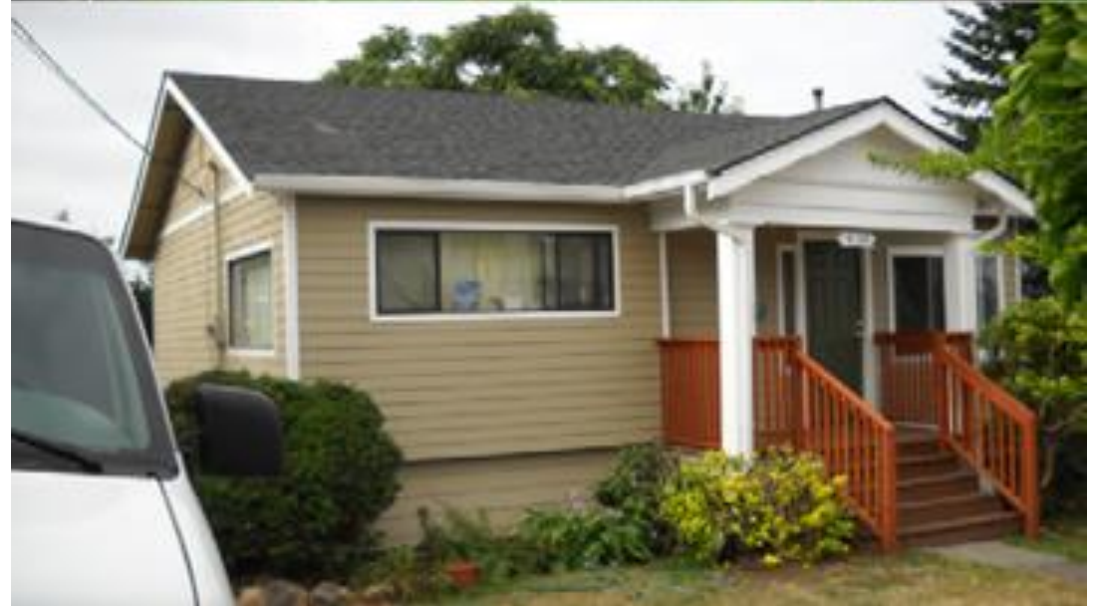
Home Repair program recipient, 2016. Before and after repairs made to home exterior.
