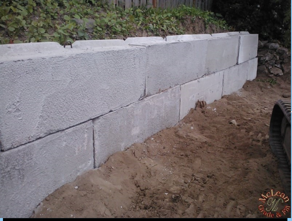
Ecology Block Wall
